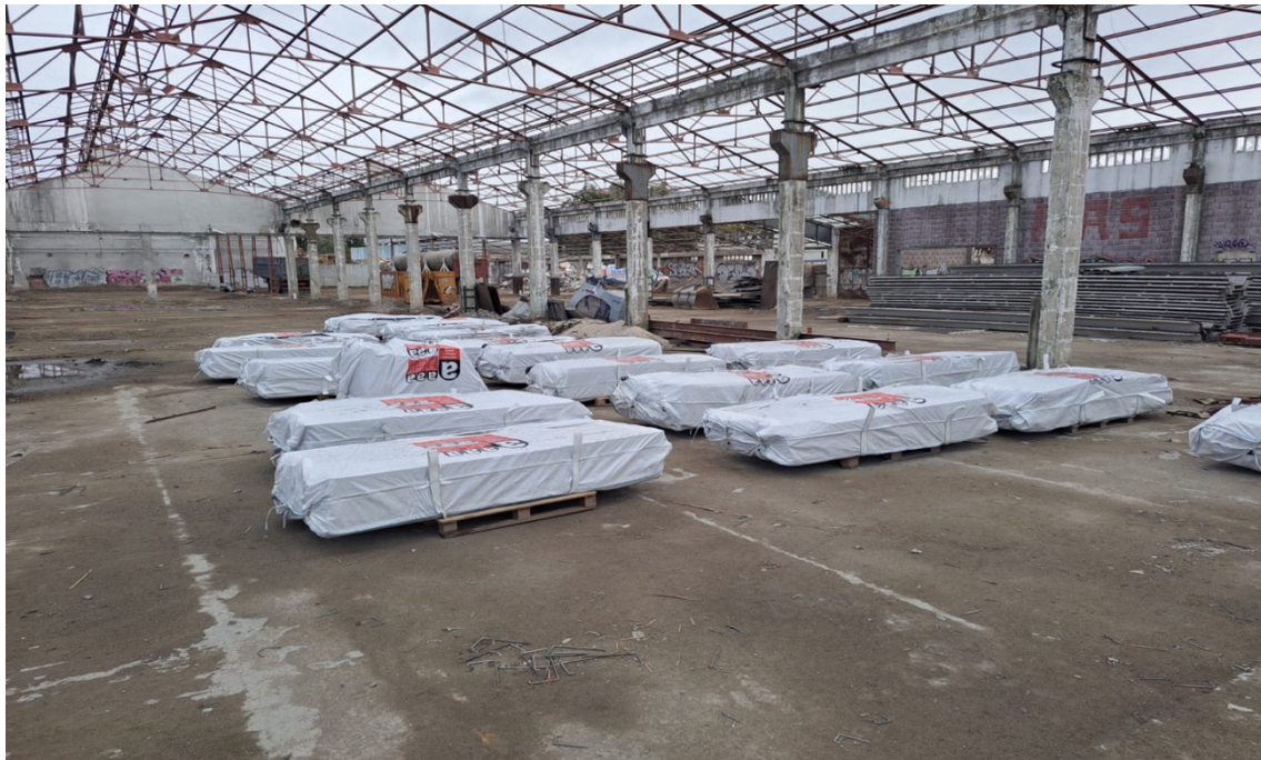
Image 1. Technical intervention on roofing with potential asbestos fibre release. Material handling requires strict safety protocols to minimize airborne exposure risk.
